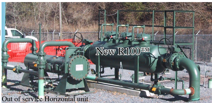
Out of service Horizontal unit
