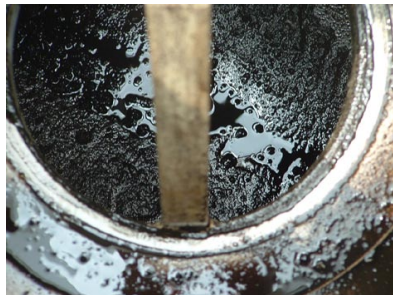
Internal dirty sump area (below element base plate).
